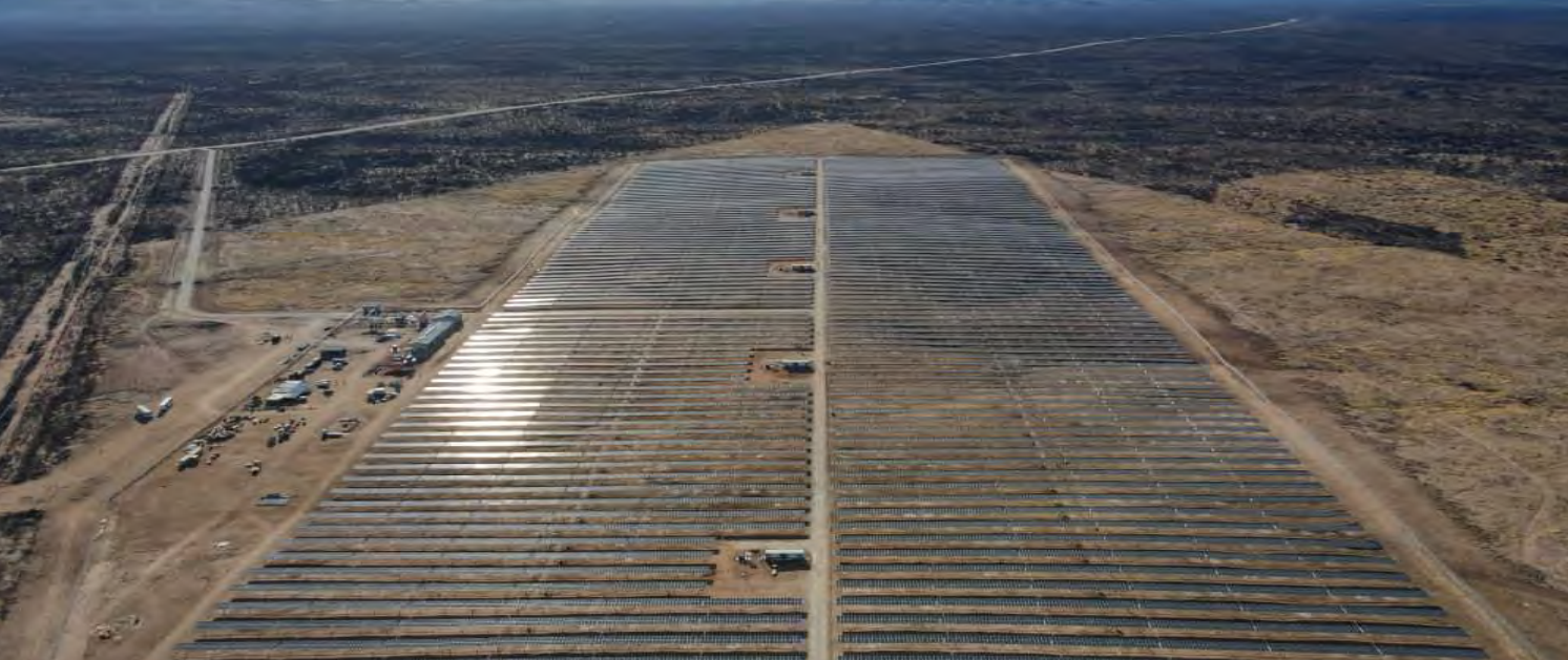
SUN POWER ... ANIREP's newly completed 20MW Omburu EPC solar PV plant
